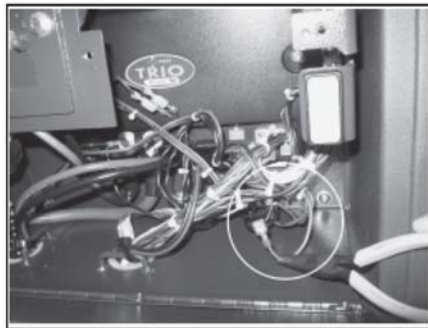
Figure 1 Jumper wire disconnected
